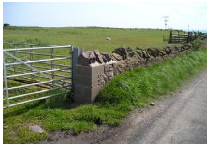
Though well constructed, the wall end repaired here would have looked more appropriate using stone rather than breeze blocks.
