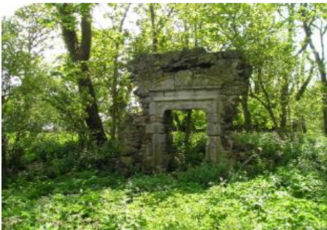
Significant old masonry features abandoned on farmland may require specialist materials and techniques to aid their repair.
