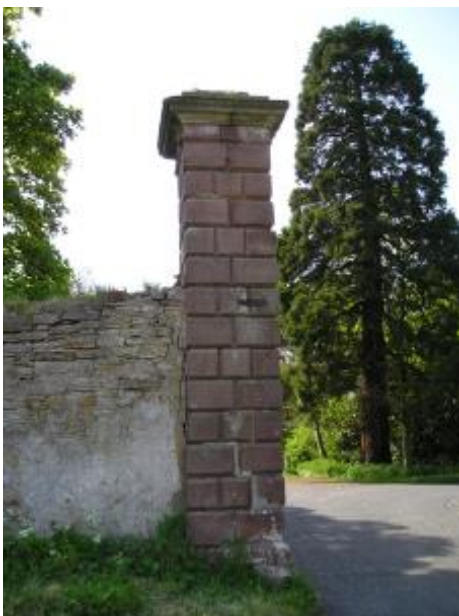
For grander residences gate piers can be quite impressive requiring more effort to maintain. Note how the wall to the left previously had a mortar render.
